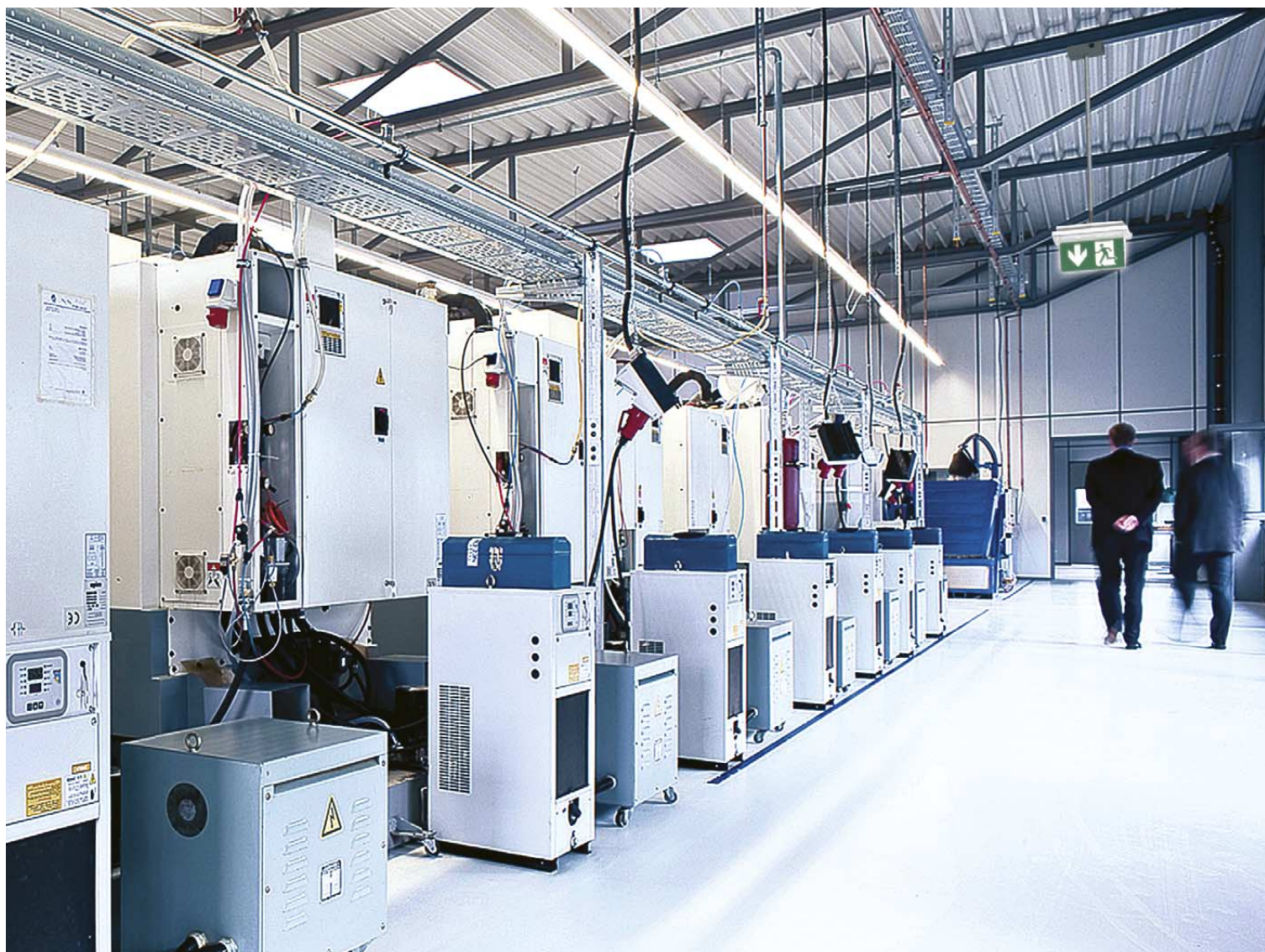
Industrial Area Emergency Lighting Application
